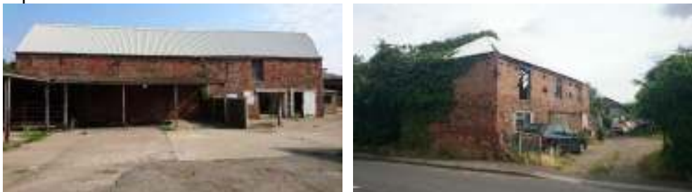
Figure 4.2: Agricultural buildings at Gibdyke Farm (left) and Northfield Farm (right), showing unsympathetic metal roofs, inappropriate alterations and in the case of the structure at Northfield Farm, visible structural defects.
