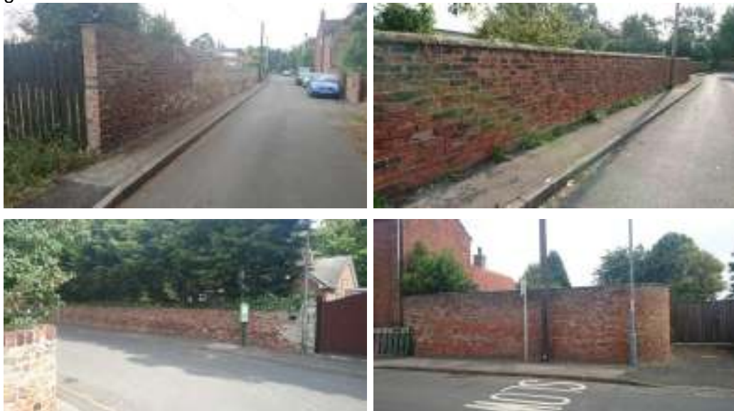
Figure 3.29: Selection of historic brick boundary walls in Misson, including along Gibdyke (top), Middle Street (bottom left) and Station Road (bottom right).
