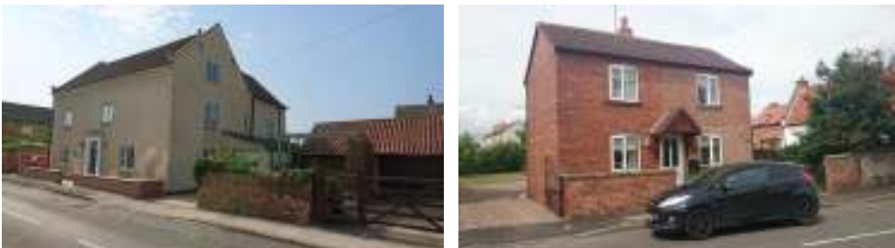
Figure 4.8: The use of standard PVC windows on the building on Middle Street (left) has resulted in the Georgian character of the building being harmed, this harm being added to by the modern render and concrete roof tiles. The PVC windows on the property on West Street (right) fail to reflect the early-19 th century architecture of the cottage and detract from its significance.
